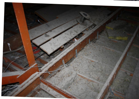
Roof space contamination.
