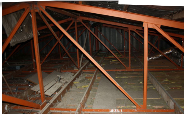
Ash covers roof trusses, beams and insulation.
